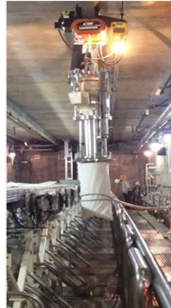
SWPF Centrifugal Contactor
